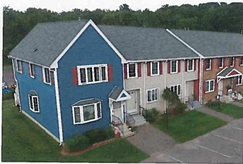
No details were left untouched during the massive renovation of Fox Meadow Condominiums, where Adam Quenneville Roofing & Siding and associates spent nearly a full year working on the envelope project.
